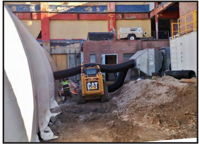
Purification Systems with carbon filtration scrub air captured under tent.
